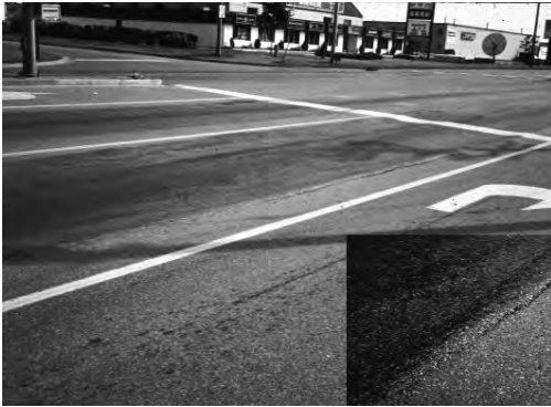
Photo 2-1: Asphalt concrete rutting of a municipal connector road conventional flexible pavement
