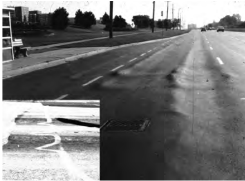
Photo 2-2: Asphalt concrete rutting of a major municipal road composite pavement
