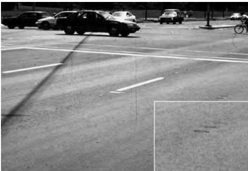
Photo 2-3: Flushing and low severity asphalt concrete rutting of a composite pavement
